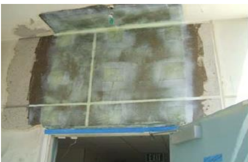
Fig.7: depict the use of advance composite in the healing of concrete spall on wall ( Chiewanichakorn & Toranzo, 2011 ).
