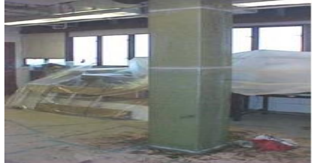
Fig.8: Depict the use of advance composite in the healing of concrete spall on wall ( Chiewanichakorn & Toranzo, 2011 ).
